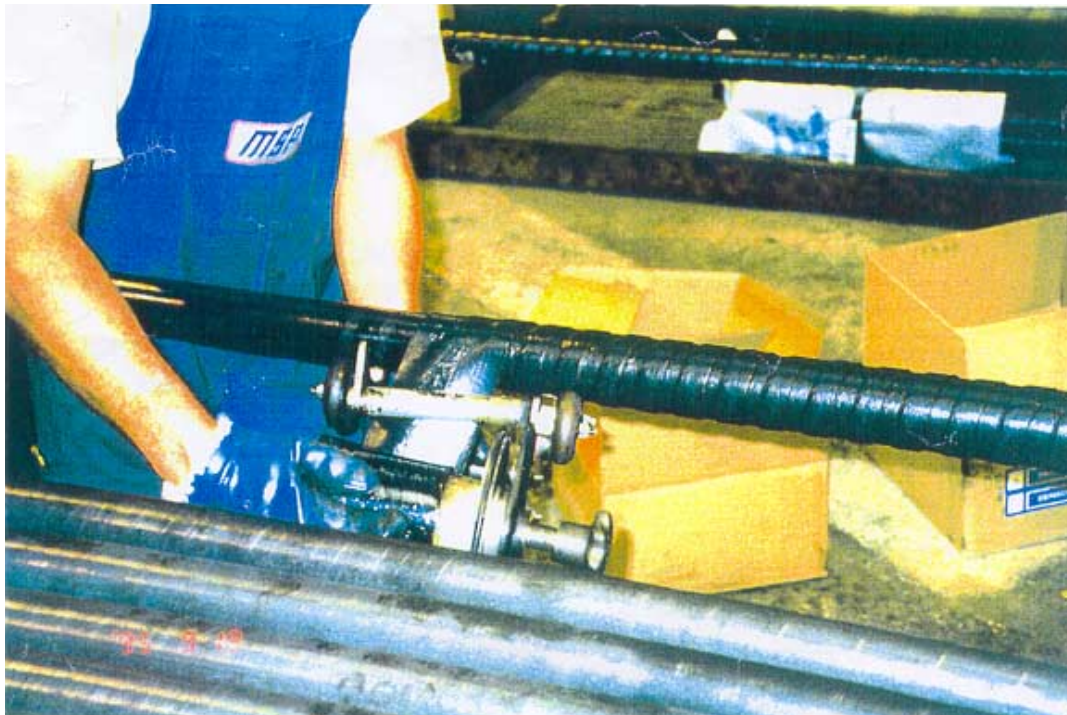
Hand Wrapping Machine used to apply Macalloy Tape to 72mm diameter Macalloy 17MHS tie bar
