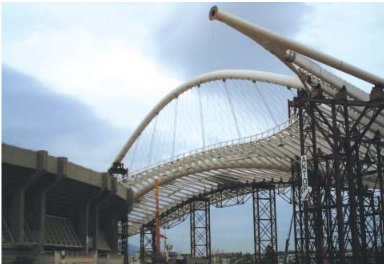
Tensoteci cable systems. Olympic Stadium, Athens
